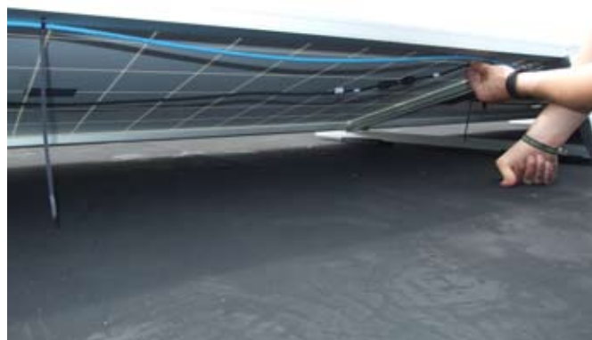
bundle home-runs with cables
